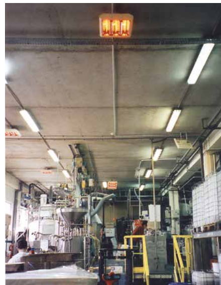
IRCF is often installed in large warehouses. They give instant and effective heat which make them profitable quickly.
